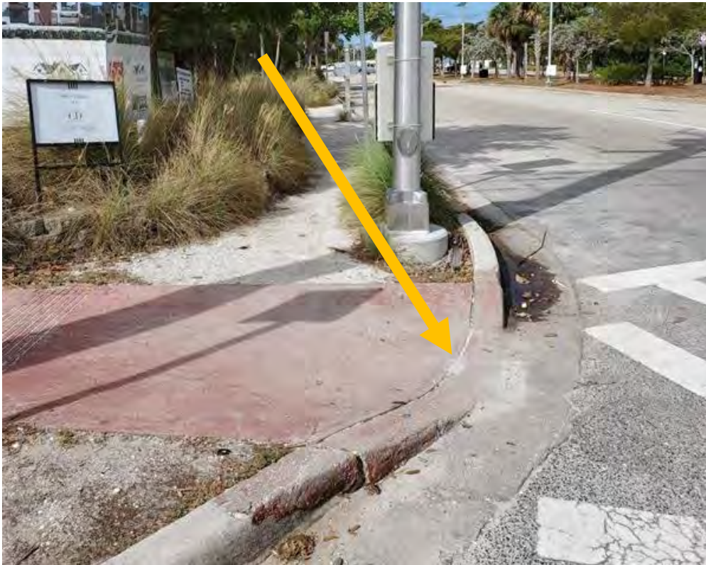
Non-compliant handicap ramps
