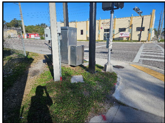
Photo 2.8. Various utilities on southwest corner of Central Avenue/10 th Street intersection, facing northwest.
