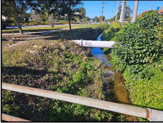
Photo 2.15. Drainage ditch running east-west along north side of 10 th Street west of Orange Avenue, facing west.
