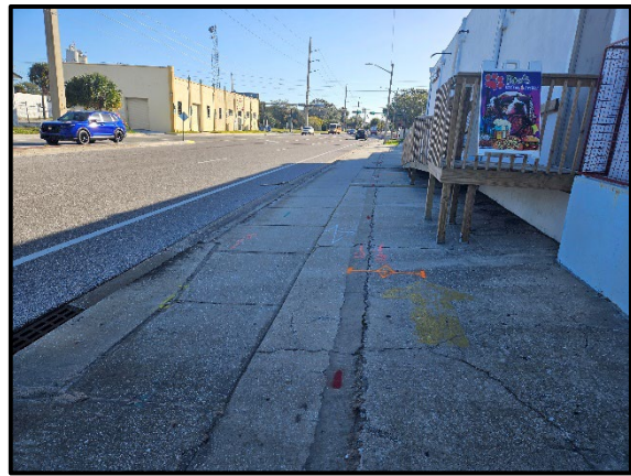
Photo 2.6. Concrete sidewalk along south side of 10 th Street east of Florida Avenue/10 th Street intersection, facing east.
