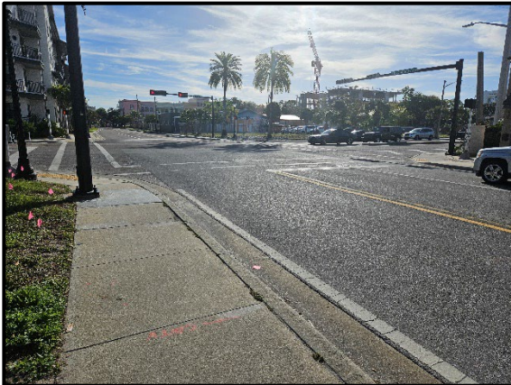
Photo 2.11. Conditions of Lemon Ave/Blvd of the Arts intersection from northwest corner, facing southeast.
