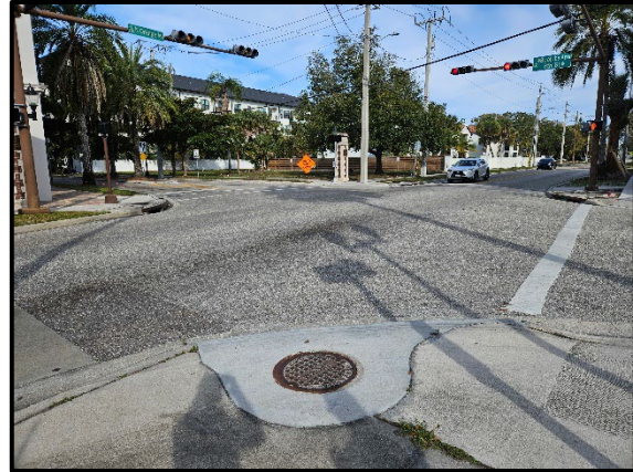
Photo 2.16. Conditions of Orange Avenue/Blvd of the Arts intersection from southeast corner across the Rosemary District, facing northwest.
