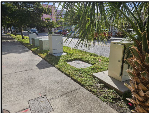
Photo 2.13. Aboveground and flagged utilities on north side of Blvd of the Arts between Lemon and Orange Avenues, facing southeast.
