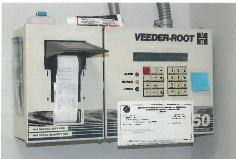
Public Works Fuel Veeder-Root Fuel Monitor
