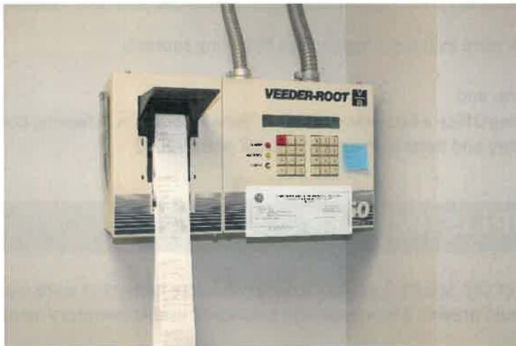
Public Works Fuel Veeder-Root Fuel Monitor
